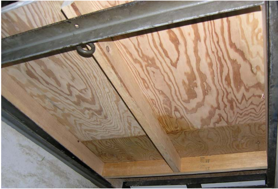
Figure B-7. Test ID BB-1. Underside of Deck at end of Test.
